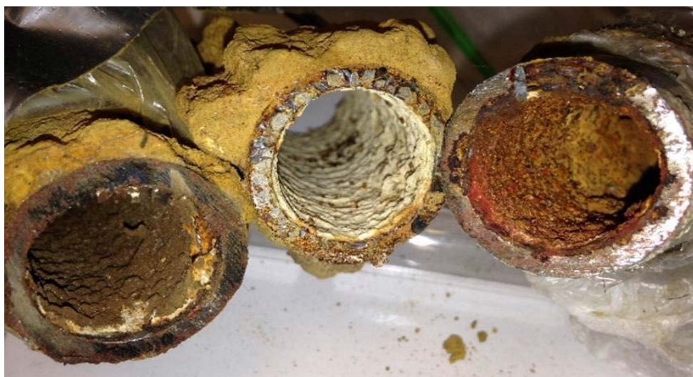
Corroded water pipes in Flint, Michigan
